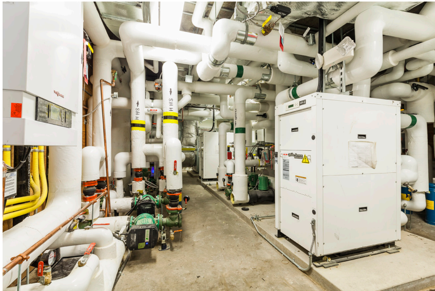
Contemporary new builds and renovations typically feature complex mechanical and electrical systems. These Guidelines and Technical Specifications provide direction for delivering appropriate service systems and building assemblies for City-owned buildings.
