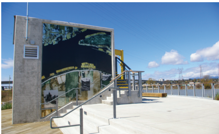
New No. 4 Road Drainage Pump Station. Graham Turnbull photograph
